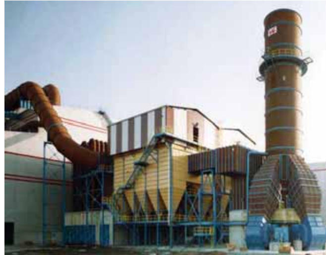
Fabripulse XLC serving an EAF in France Flow: 1,600,000 m 3 /h upgrade to 2,200,000 m 3 /h
