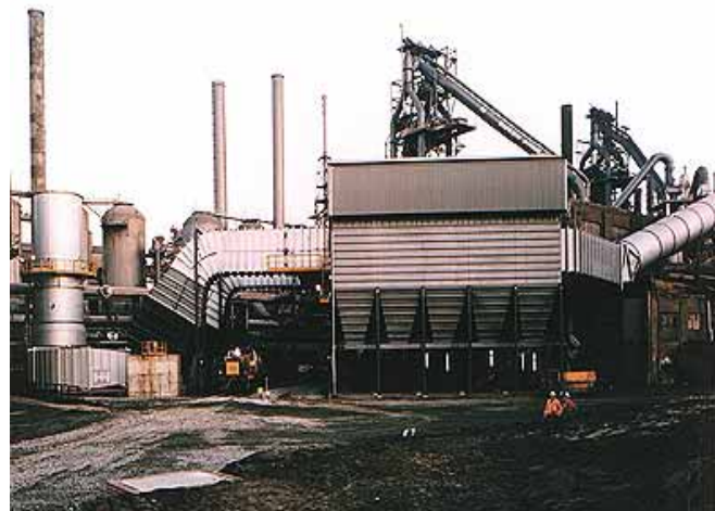
Fabricpulse XLC serving two BF cast houses in England Flow: 492,000 m 3 /h
