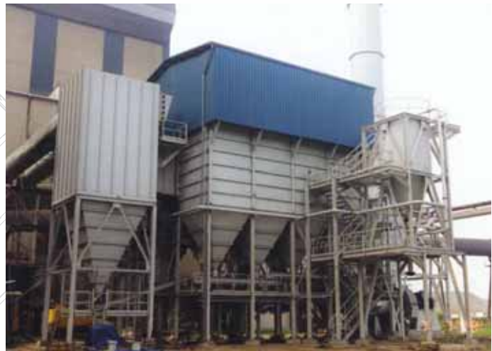
Fabripulse XLC serving an iron desulphurisation in Netherlands Flow: 300,00 m 3 /h
