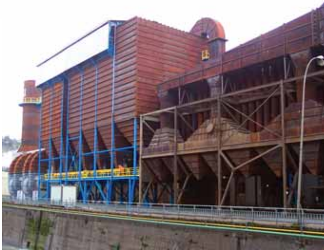
Fabripulse XLC serving an EAF in Spain Flow: 2,000,000 m 3 /h
