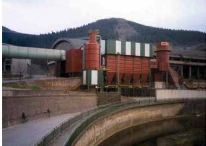
Fabripulse XLC serving an EAF in Spain. Flow: 1,500,000 m 3 /h
